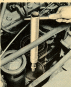
Fig. 2. Oil-line leaks on your 3-cyl model can maybe be eliminated by using this tool.
